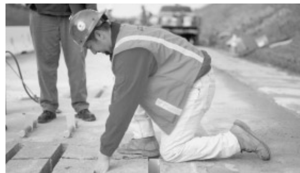
A technician installing a steel dowel bar in a section of U.S. 101 near Ukiah, CA that is being retrofitted
